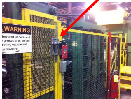
Interlock Mounted on Enclosure Gate
