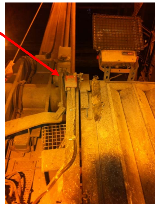
Converter Maintenance Lift
